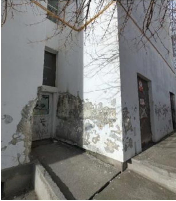
Photo 10 – The exterior walls show dampness
