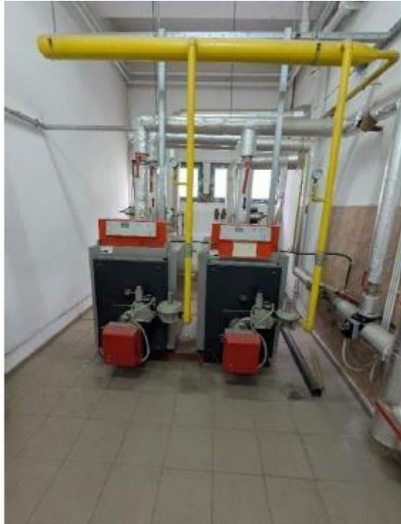
Photo 7 – Photo of the thermal plant, one can observe the two boilers providing heating and hot running water preparation
