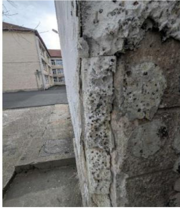
Photo 11 – The current thermal insulation is in a very advanced degradation condition
